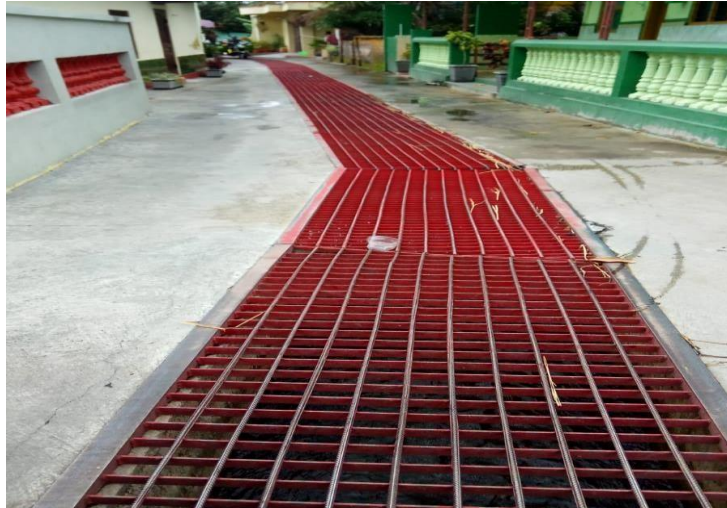
Figure 5. Sewer in Ponggok Village
